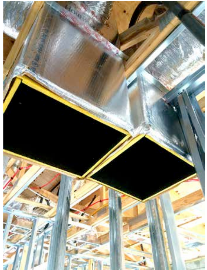
Photograph 9: Rigid Duct —Go with rigid duct as it is much easier to seal where it penetrates ceilings.
