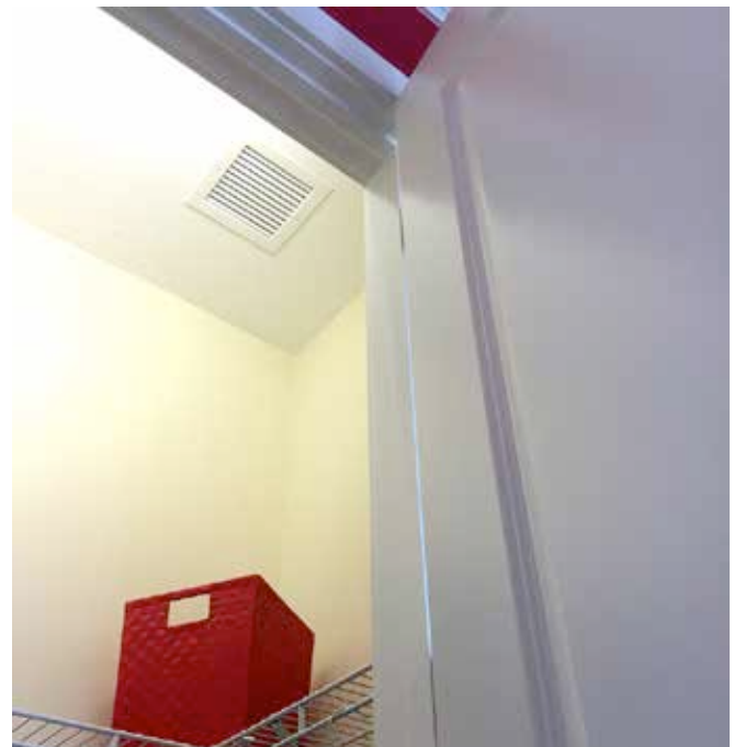
Photograph 12: Closets Need Returns —What spaces have the least load? Closets. Closets need “active” returns at the ceilings and undercut doors. Closets are now getting colder.
