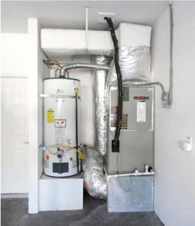
Photograph 2: Air Handler in Garages —There are complications. See Kevorkian. The air in an attic and garage comes from the same place...outside. Same dew point but higher relative humidity. It gets worse...wait for it...in a hot attic the box that makes air cold is actually warmer. Not so much in a garage. Air handlers themselves are colder as are the supply plenums that are attached to them. So stuff sweats more...way more. We actually increased moisture problems with equipment and ductwork when we moved air handlers from attics into garages.
