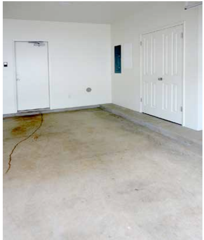
Photograph 3: Air Handler in Closet in Garage — Easy peasy right? Not if they are also gas furnaces. What about combustion air?
