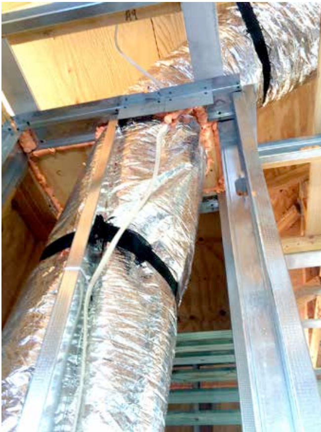
Photograph 8: Flex Duct —The mechanical closet is going to be slightly negative. The ductwork penetrating the ceiling needs to be sealed in an airtight manner if the ceiling is at the underside of a vented attic. You do not want to pull hot humid air down into the mechanical closet from the attic. The supply and return ductwork should not be flex duct as it is extremely difficult to seal.
