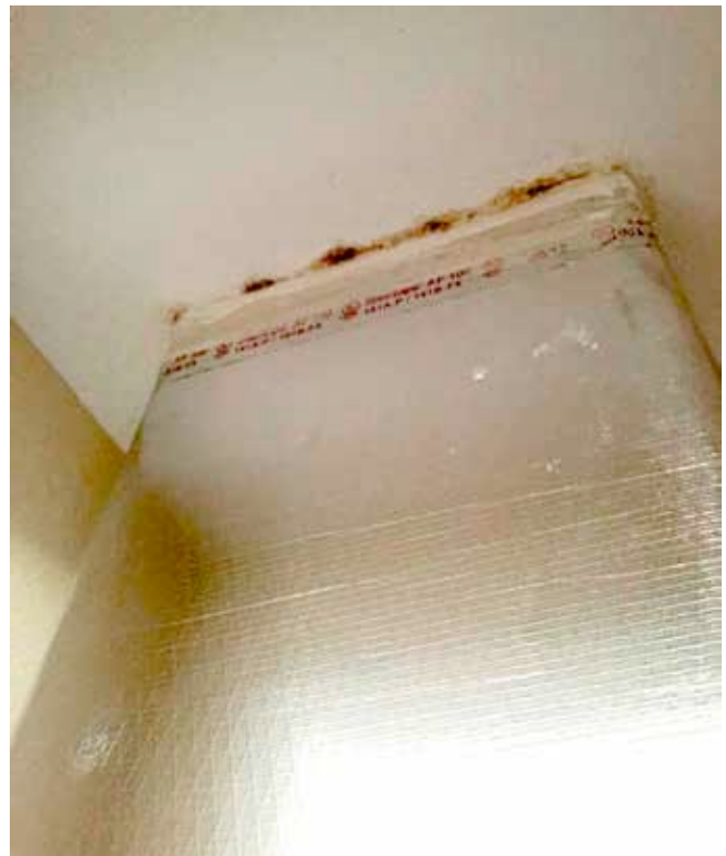
Photograph 7: Mold at Ceiling of Mechanical Closet —If all you do is put the air handler inside the house in a closet inside the house you will get mold. Not a lot. But some. It typically ends up at the ceiling of the closet where the supply plenum penetrates the ceiling. This problem goes away with a grille on the return plenum (see Figure 1 again) coupled with a jump duct or transfer grille.
