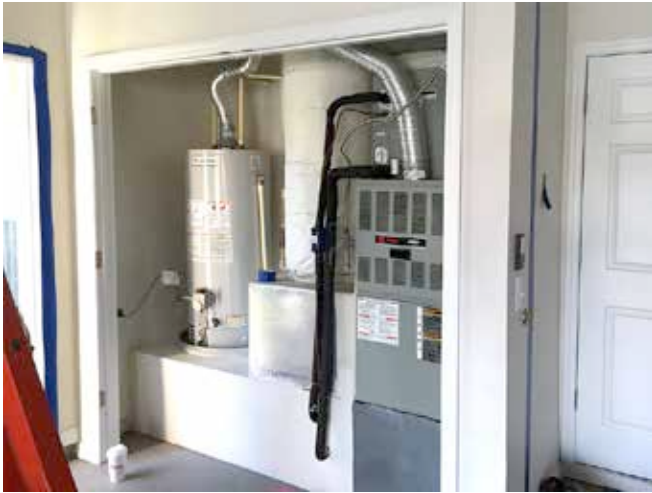
Photograph 4: Gas Water Heater and Gas Furnace In Closet— Standard gas water heaters and gas furnaces need combustion air—basically a big hole connecting the closet to the garage. Defeats the purpose which was to stop the sweating.
