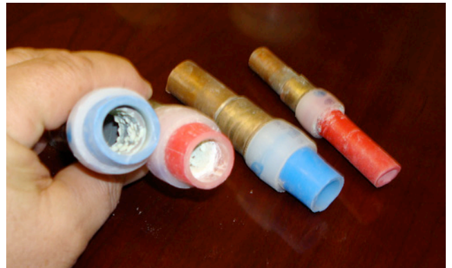
Photograph 5: Meringue Dezincification— Note the corrosion product, zinc oxide residue, blocking the fitting.
