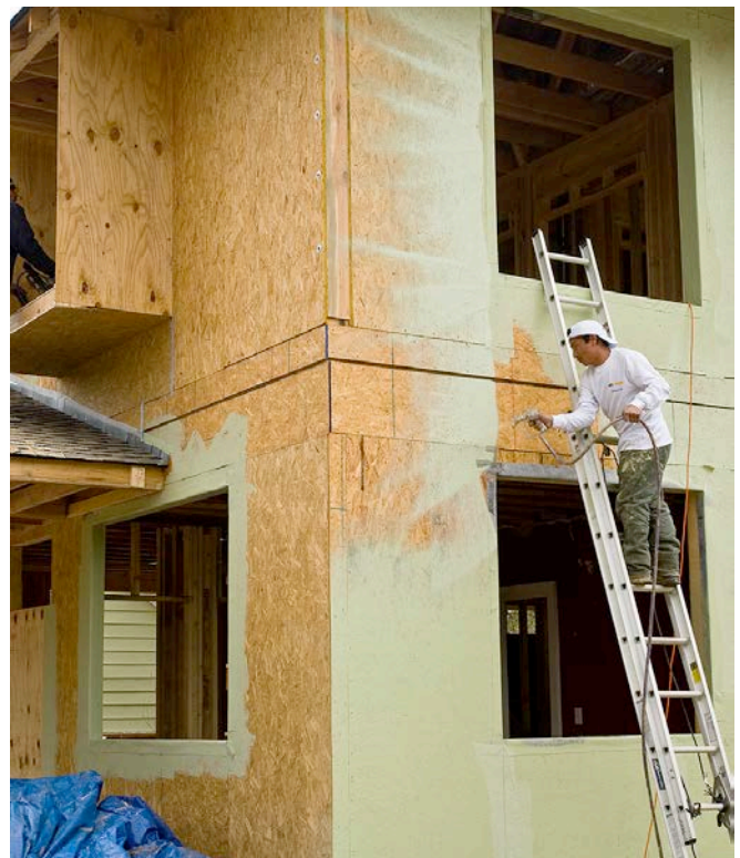
Photograph 9: Fluid Applied Air Barrier —The coatings needed to be able to span joints and they needed to be vapor permeable. And their most important function, rainwater control could not be compromised.
