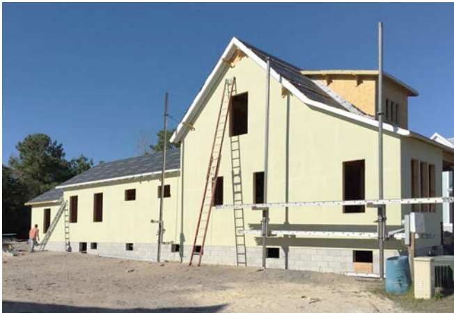
Photograph 10: Water Control/Air Control Continuity— The fluid applied coating must connect to the air control layer of the roof assembly and to the air control layer of the foundation assembly.
