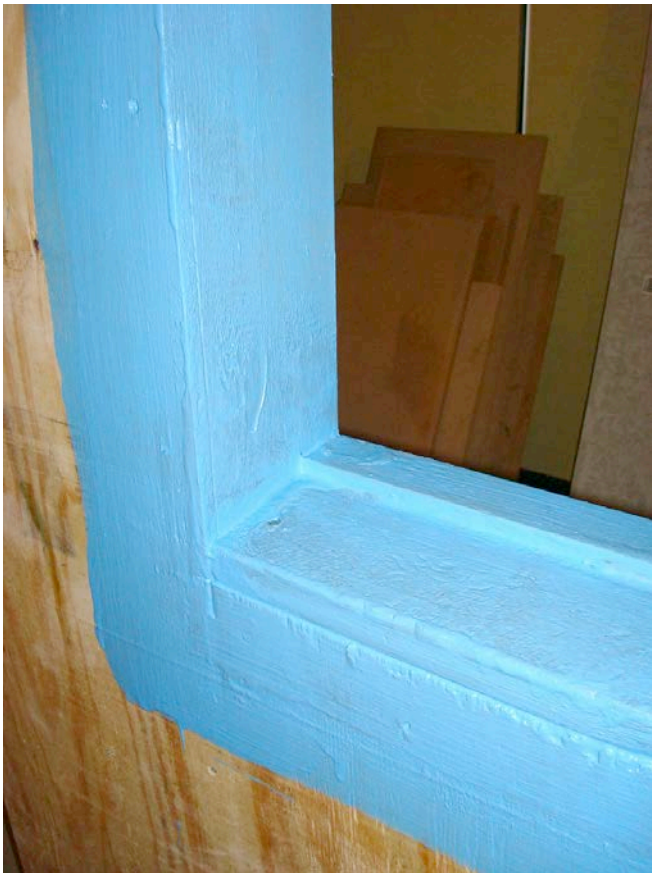
Photograph 11: Window Opening— Origami is not a necessary skill with fluid applied flashing systems.
