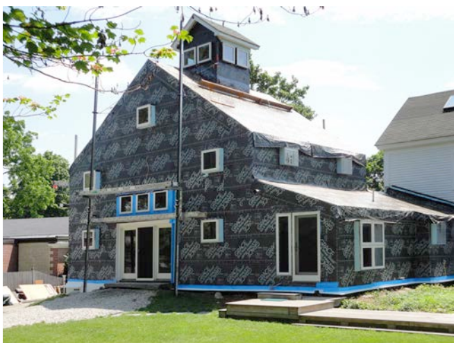
Photograph 8: Fully Adhered Membrane —Ultra high levels of airtightness with ultra high levels of cost. Not the easiest stuff to install either. I should know, this is my place.
