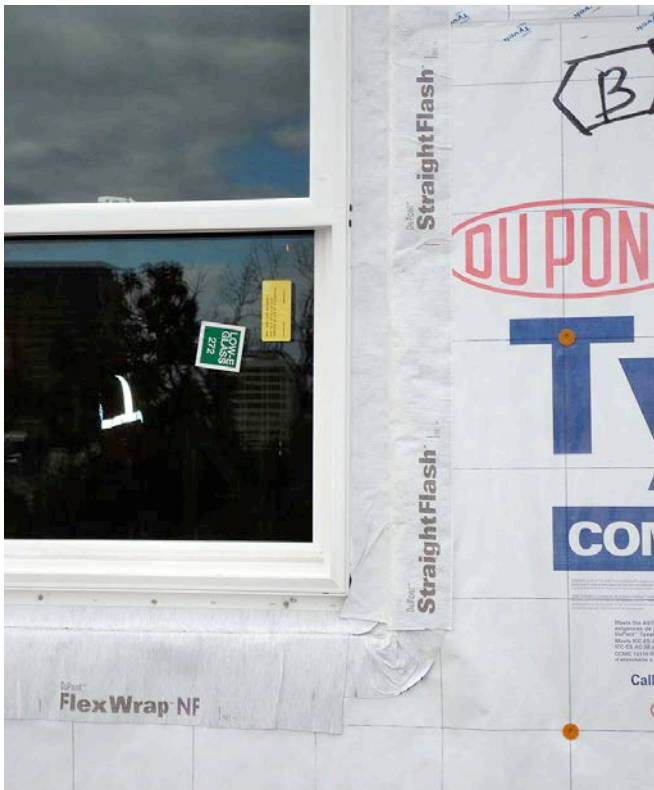
Photograph 6: Robust Rainwater Control —Numerous elegant and clever accessories were introduced to deal with rainwater control particularly at window-to-wall interfaces. This is a formable and flexible membrane “pan flashing” system.
