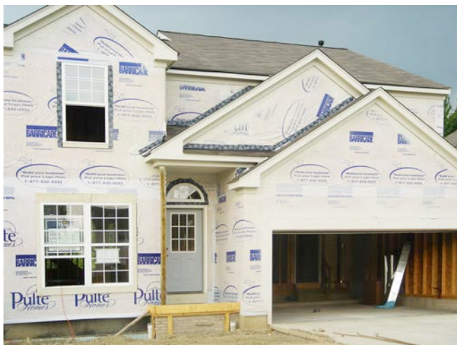
Photograph 5: Air Infiltration Barrier —Classic housewrap rainwater control layer and air control layer. Note the beautiful job of flashing integration with the housewrap. The outside is the right place for air control.
