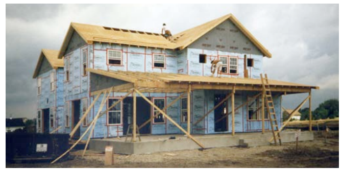
Photograph 14: Insulating Sheathing Water and Air Control Layer— The insulating sheathing provides three functions in this approach – water control, air control and thermal control.
