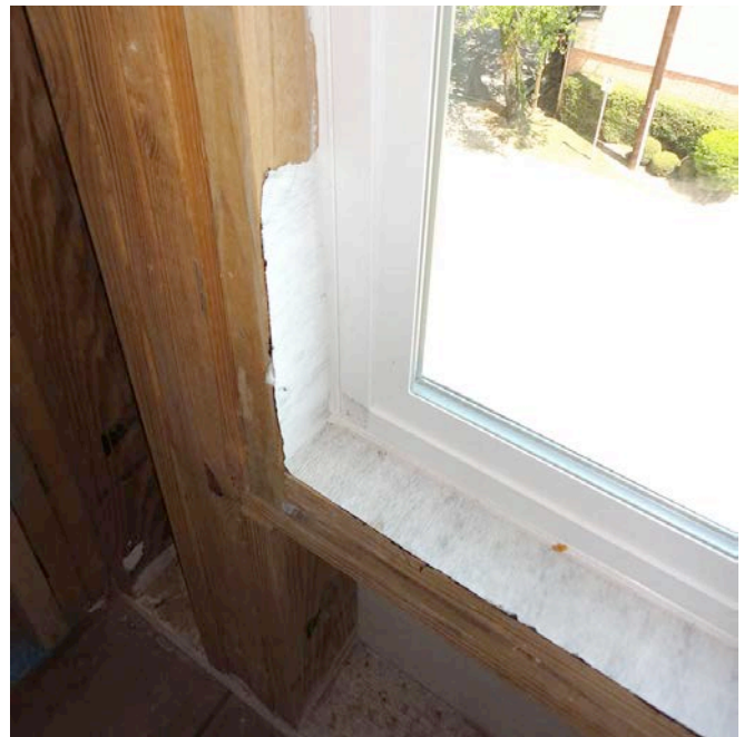
Photograph 7: More Robust Rainwater Control —Beautiful “under window gutter” where the pan flashing is sealed to the interior of the window unit for air barrier continuity.
